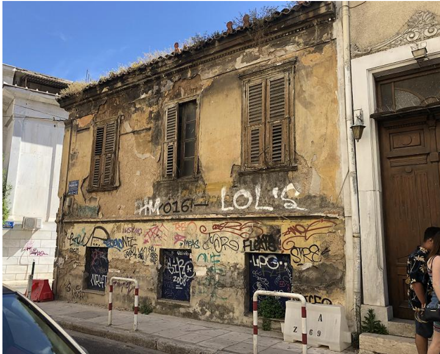
2.2 Typically defaced building, central Athens, Greece, May 2019.
