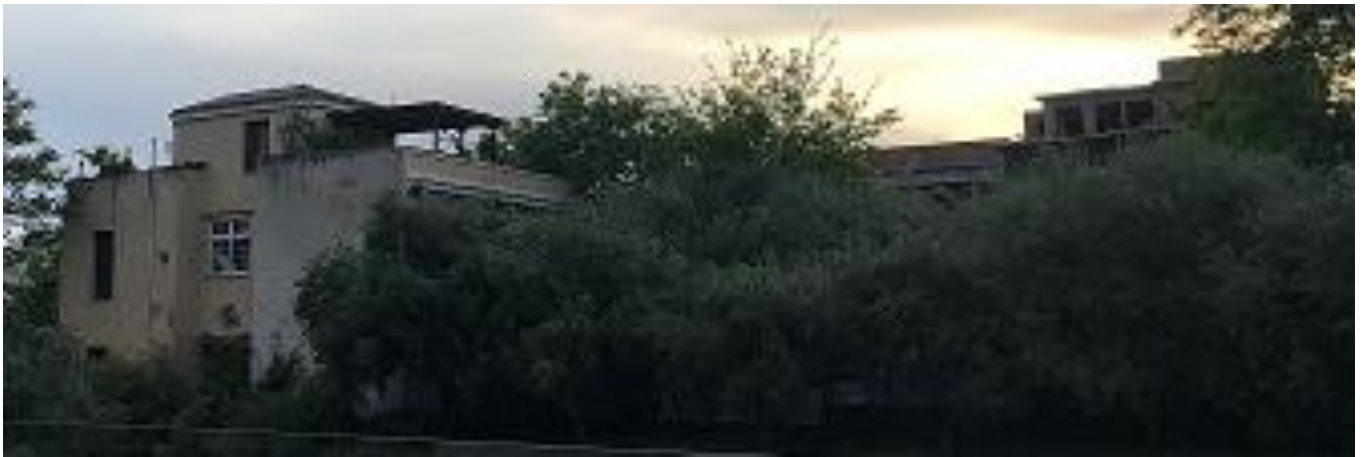
3.13a Detail of buildings with unscreened openings visible from the forecourt of the NAM, Athens, May 2019.
